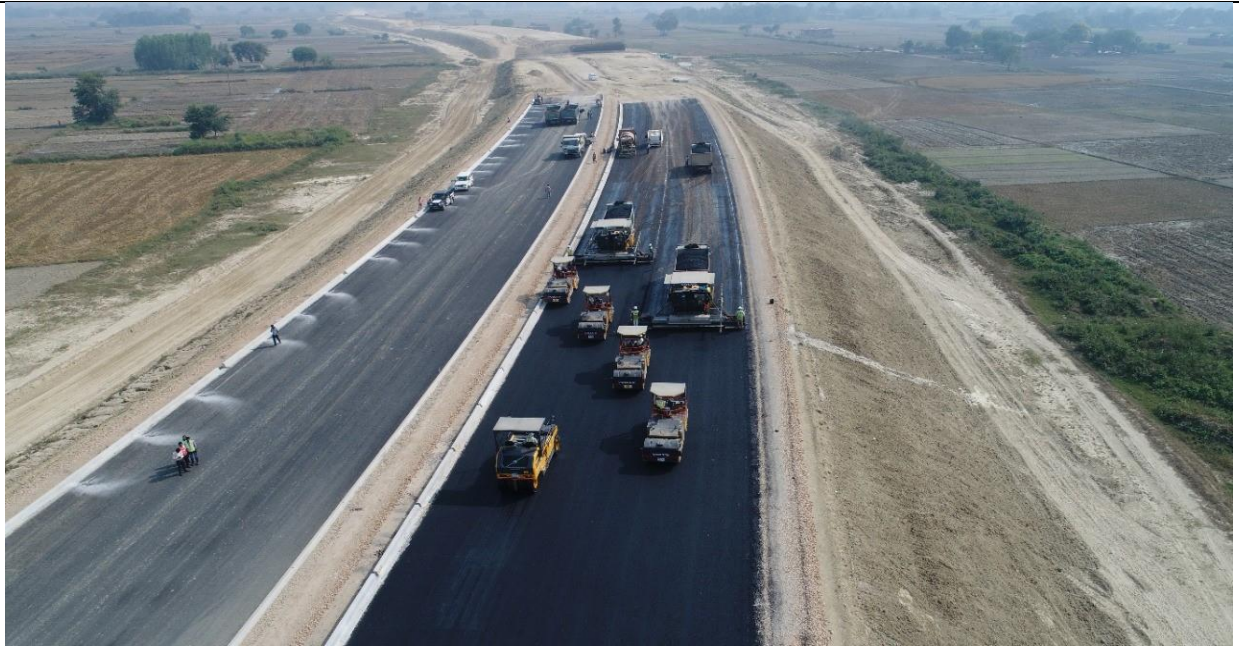
Project Management Consultant cum External Technical Auditor: Laying of Bituminous Surfacing; (Access Controlled Purvanchal Expressway, 6-lane with Paved Shoulders, Green Field), Uttar Pradesh
