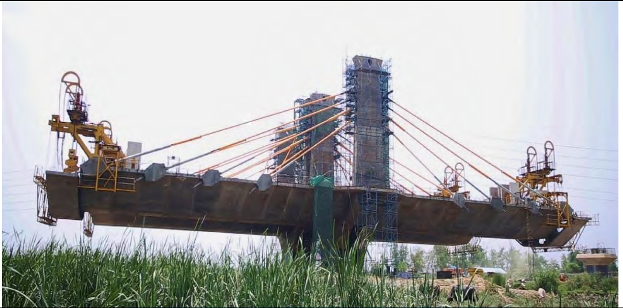
Third Party Inspection & Quality Audit: Stay Cable Work , Elevated Road MayurVihar - Yamuna Bank Section (6-lane), Barapullaha Phase-3, Delhi
