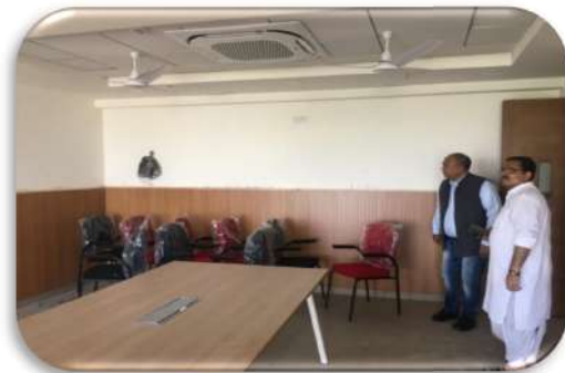
Installation of CCTV ,Furniture, Doors in Vivekananda Institute of Values in Gurgaon, Haryana
