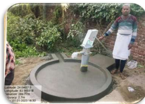
Hand-pumps in Palamu and Garhwa District of Jharkhand.
